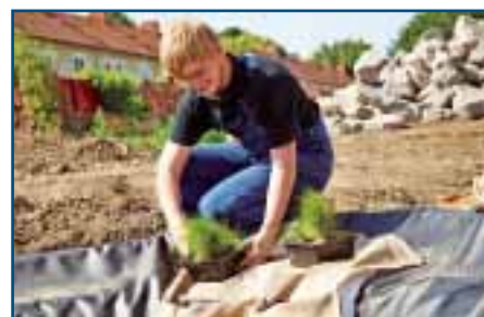
8. Planting on steep areas Steeper sections are planted using marginal plant holders. Use large rocks to first weigh the plant holders down so that you can insert the plants.
