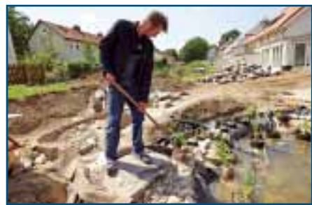
10. Gravel and water After the gravel, at last it is time to put water in the pond: first fill it half full, and then after the liner has completely settled, fill the pond completely.
